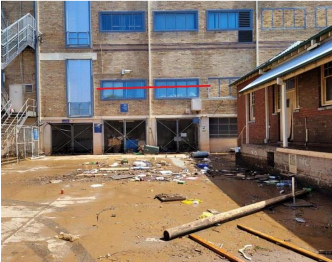
Telstra's Lismore exchange showing height of flood
